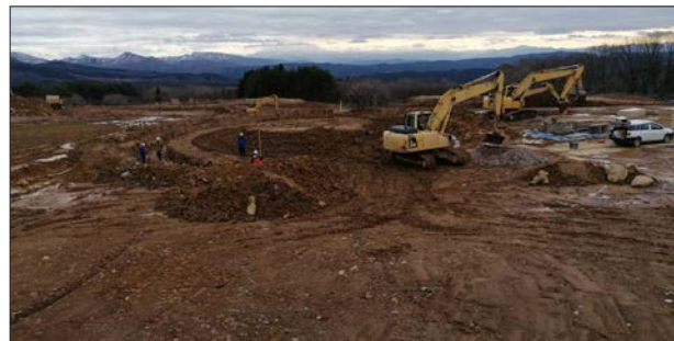
In Sakata on the main island of Honshu, cowsheds are currently being built in addition to the biogas plant. This location should be ready in autumn 2021.
