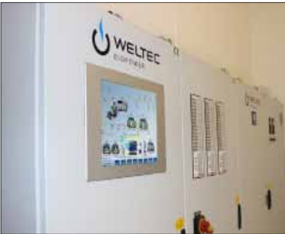
In South Korea, the optimum function of the components will be controlled by the PLC-based LoMOS control, which is custom-developed by WELTEC.
