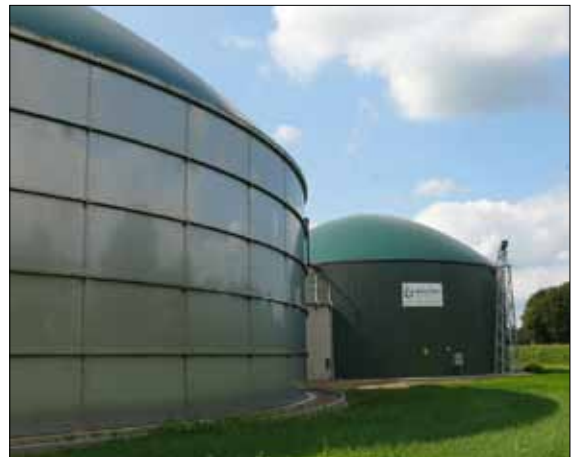
Starting from the early summer of 2016, the operator will supply the stainless-steel digester with its capacity of almost 4,000 m 3 with 100 tons of organic waste a day, whereof 70 % are pig manure.
