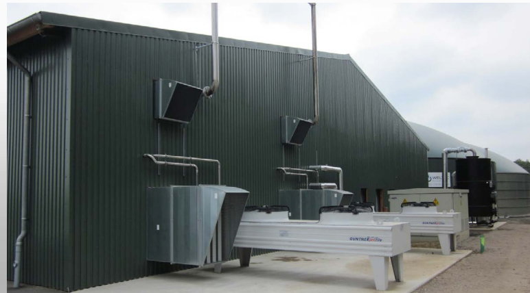
The heat is partly used to dry the digestate.
